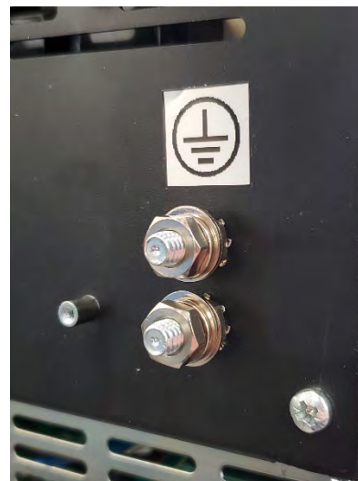
Figure 7A: External Earth Termination
